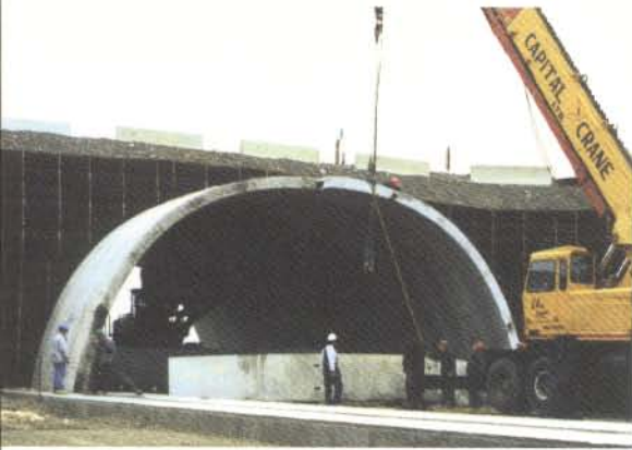
👂 Temporary Terratrel wall supported "Stage 1" diversion allowing uninterrupted traffic during bridge dismantling.
